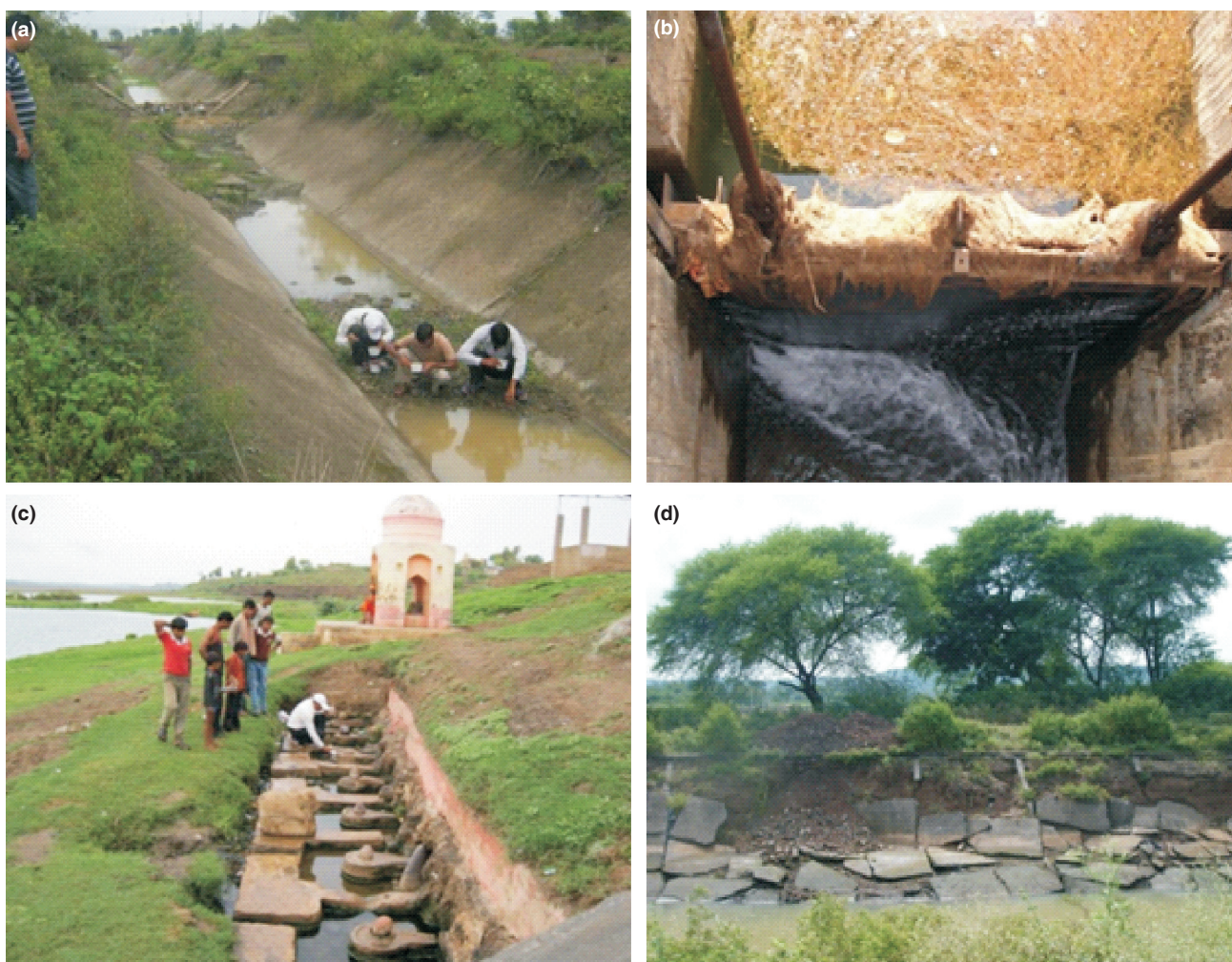
Photographs showing: (a) water stagnation in canal, (b) stagnation at gates, (c) breeding sites at religious places, and (d) broken margins of canal.
